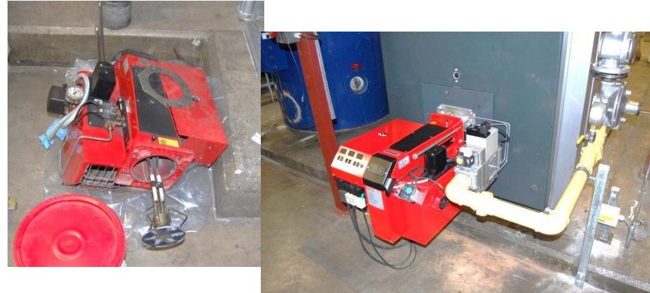
LPHW Burner Switch
