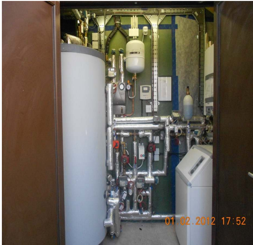
PLANTROOM: Accumulator on left, heat pump and boiler on right, solar equipment upper centre
